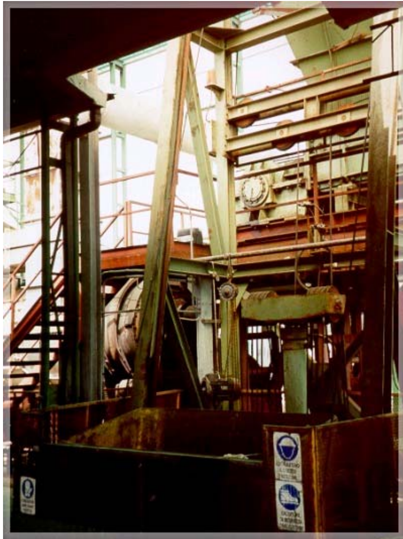
Figure 5. Waste Loading Point: Hopper, Feeder, Grinder
