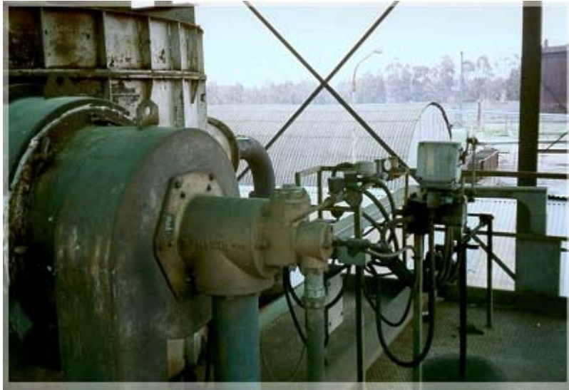
Figure 8. Combustion Chamber: Burner
